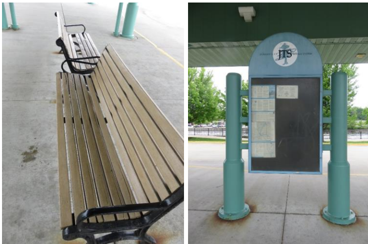
At downtown Transfer Center, benches need replacement and footings are rusting.
