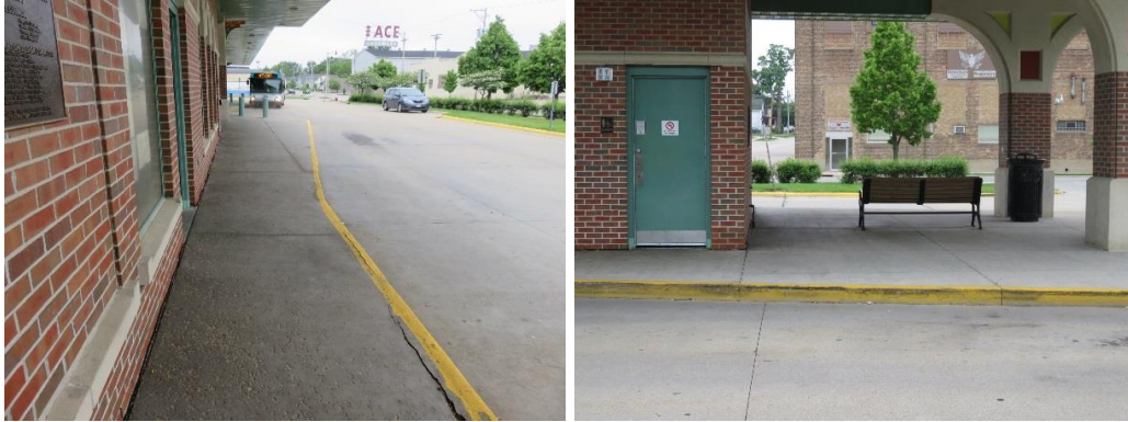
East Milwaukee Street stop has 48-inch clearance. BJE buses stop near bench for clearance.
