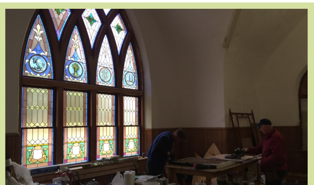
The Friends of Oak Hill Chapel made substantial progress on chapel restoration.
