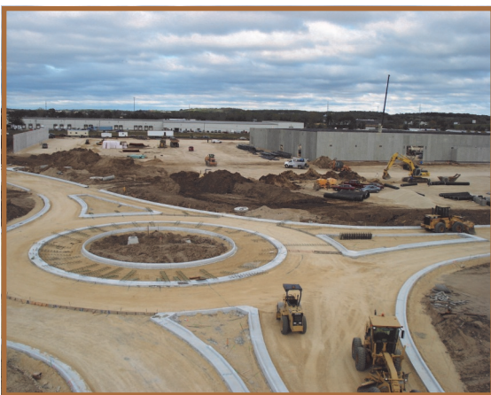
Pictured above is the new roundabout under construction on Morse Street. Construction is expected to be completed in the Fall of 2007.
